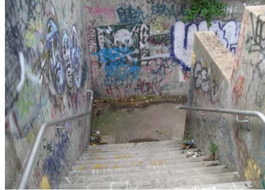
Figure 38 Socially-unsafe and disability non-compliant access to the Yarra rail and foot bridge on the northern (City of Yarra) side
