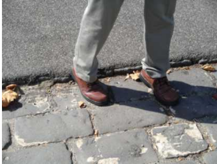
Figure 17 Disability non-compliant crossing - Michael Street
