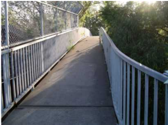
Figure 1 The non-DDA compliant overpass of Hoddle Street at Vere Street
