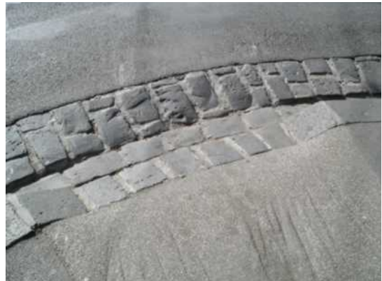
Figure 2 Non-DDA compliant kerb ramps on the South side of Smith Street
